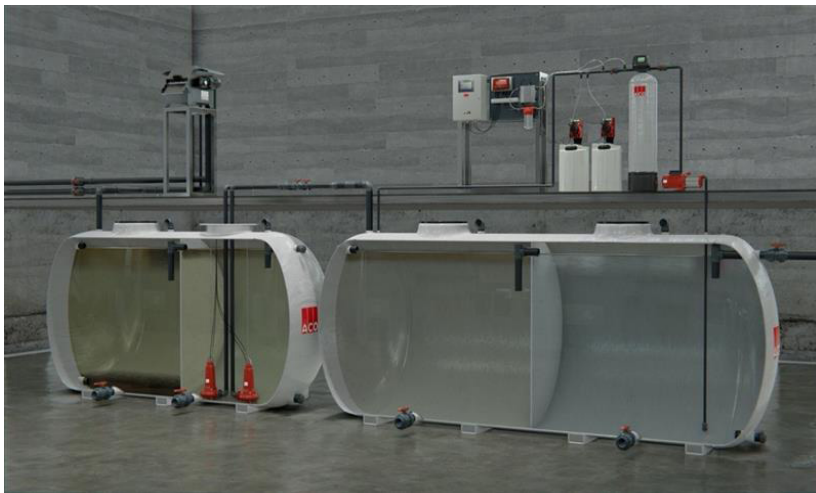
Rainwater collection tanks and cisterns
